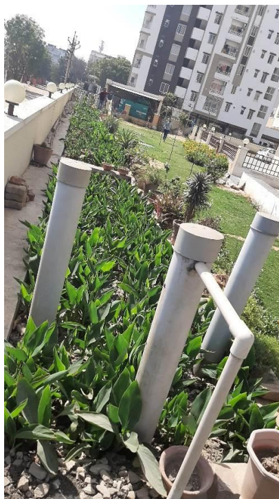
Constructed Wetland for treatment of domestic wastewater from residential area (NIH Colony Roorkee)
